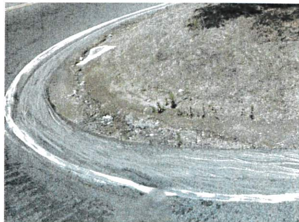
Figure 12: Evidence of Truck or Vehicle Scraping
